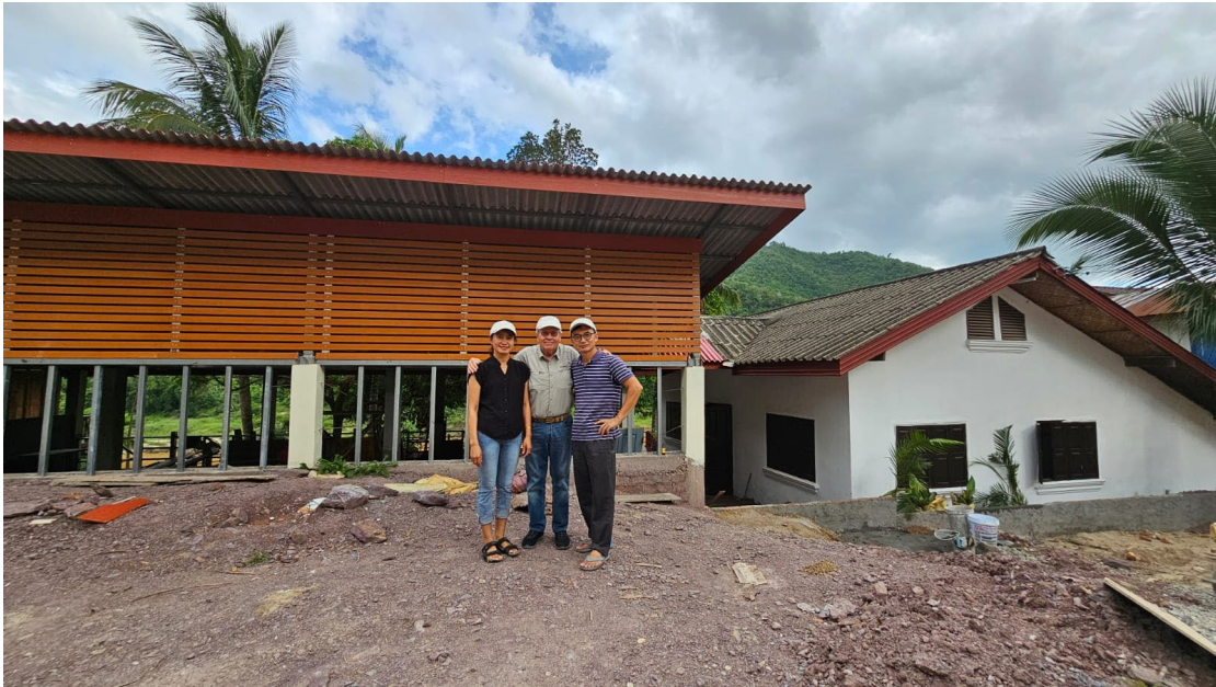
Dr. Phetsamone, Dr. Luc and Ms. Khamman are supervising construction of a new eye care facility in Pakbeng District
